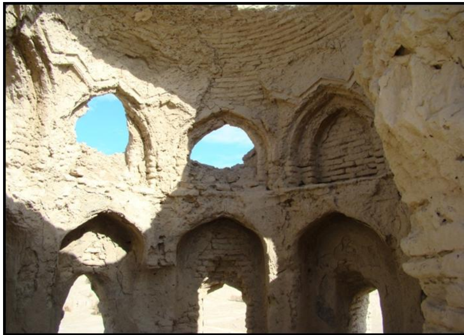
Figure 9. Zahedan-e Kohneh: interior view of one of the rooms on the third floor of the tower in the northwest corner of the castle (by the authors).
