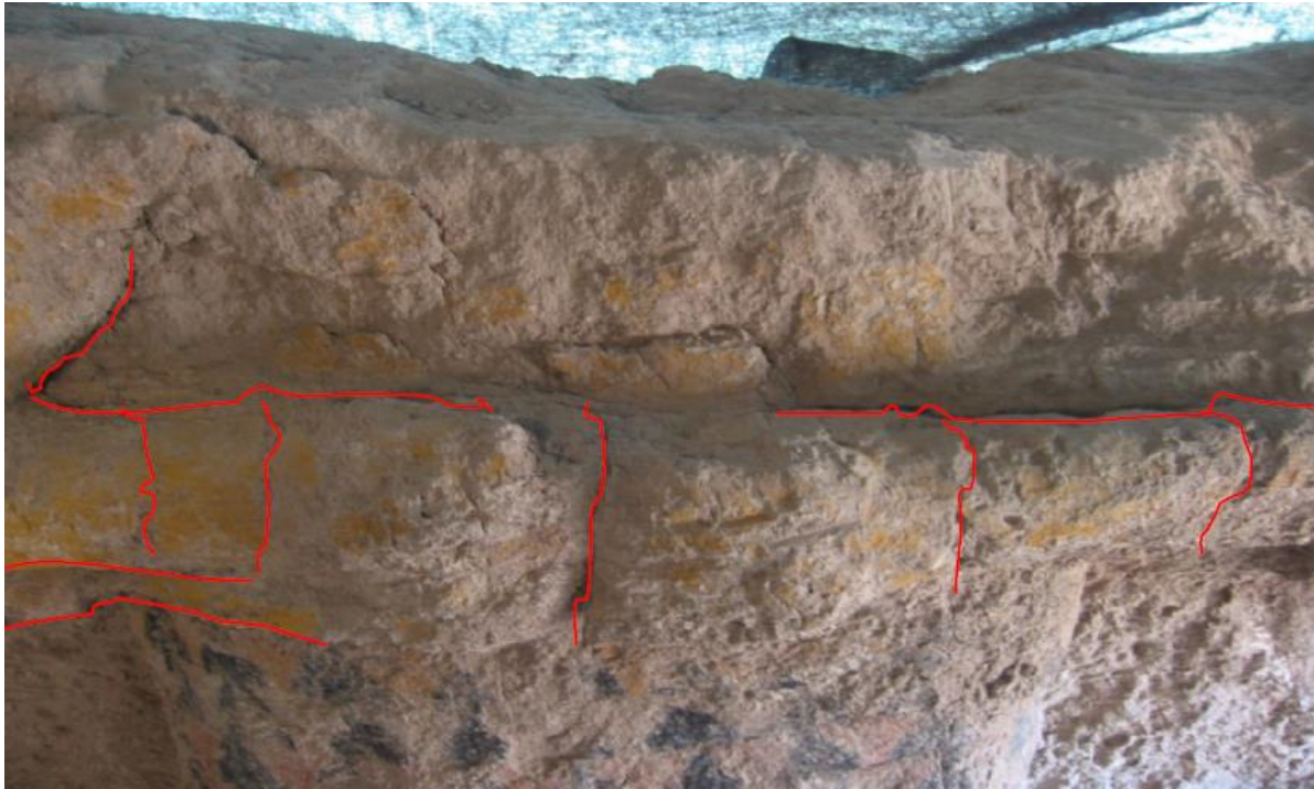
Fig. 9. Parallel cracks in forearm of statue and separation of chest and waist scarf due to wet to dry contraction of clay mud (author, 2006).
